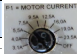
Figure: P1 of a 7.5 kW motor starter
